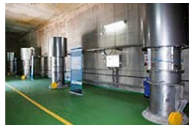
Turbines of the Mutriku OWC plant
