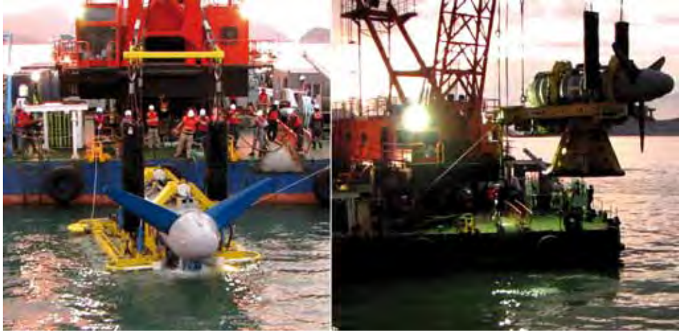
▲ Installation of HyTide 110-5.3 of Voith Hydro
