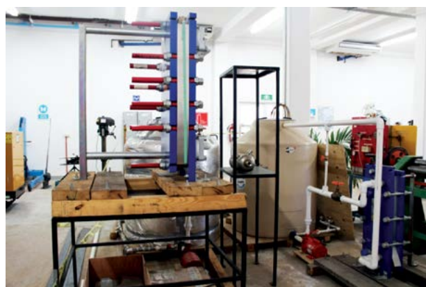
OTEC facility at CEMIE-Oceano
