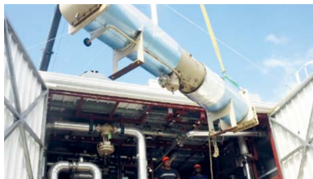
Test bench facilities La Réunion Island
