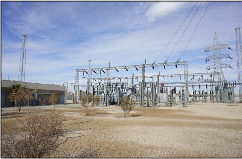
Figure 7: Typical 33/132kV Substation
