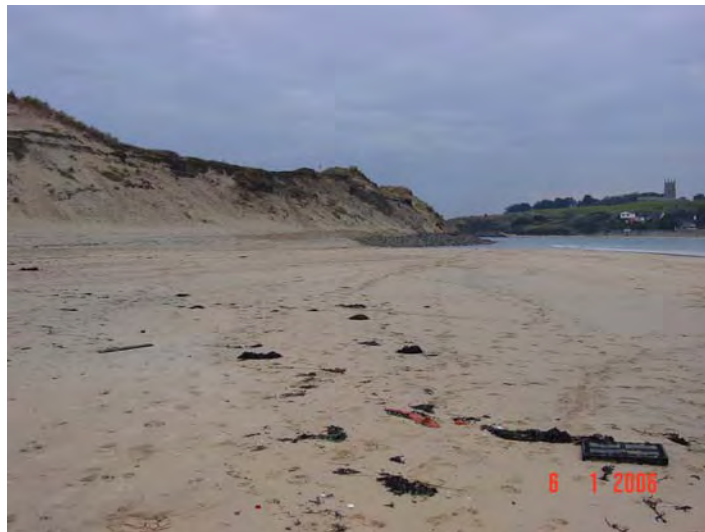
Plate 7.8: Looking towards Harvey's Towans dunes and Hayle Estuary mouth from the beach. Note rock revetment at the toe of the dunes in the distance and the exposed tipped material (January 2006)
