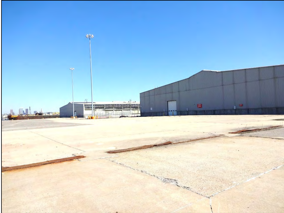
Looking southwest toward existing building structures at SBMT (39th Street "Pier"). SBMT has been determined not eligible for listing in the National Register. Structures and paving will be removed, and the area will be repaved.
