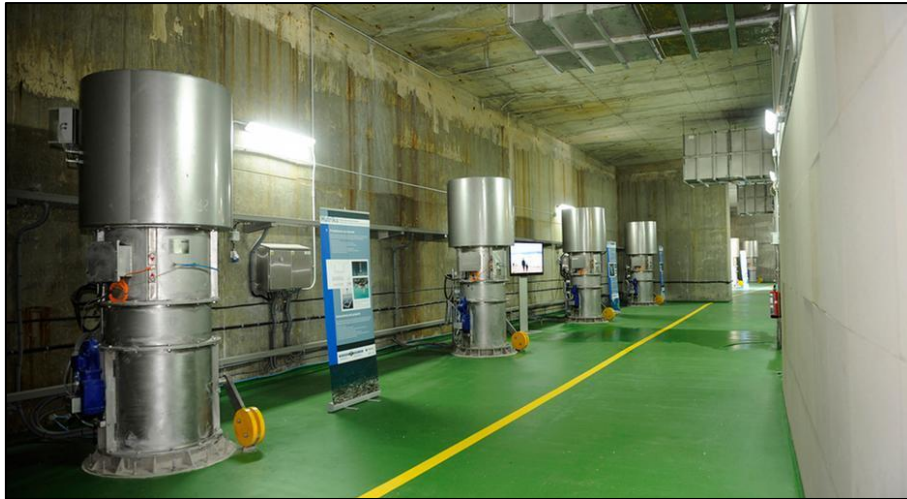
Figure 6. Mutriku Wave Power Plant turbines inside the plant.
