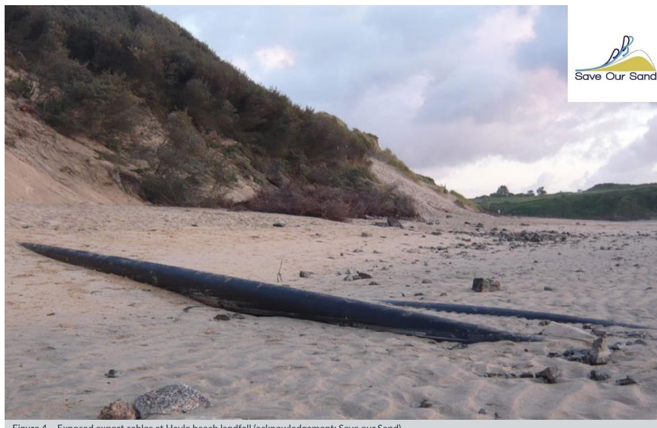
Figure 4 – Exposed export cables at Hayle beach landfall (acknowledgement; Save our Sand)
