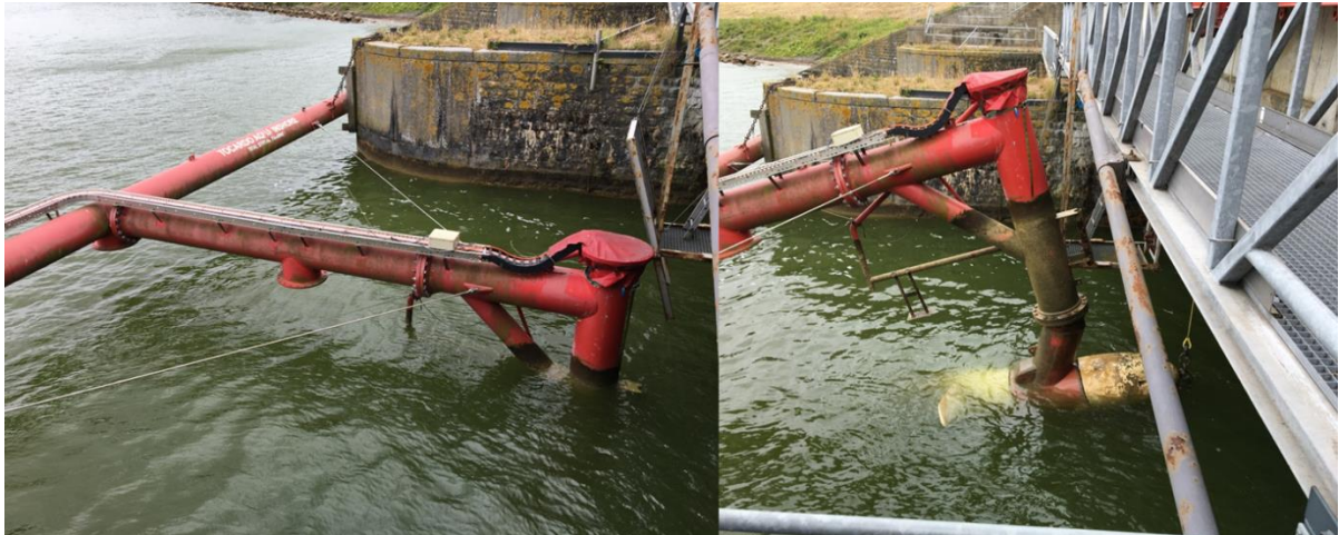
Figure 3.5. The beam construction holding the Tocardo T1 tidal turbine in sluice 2 of Den Oever that was used to serve as a base for developing a robust housing construction to perform DIDSON measurements here.
