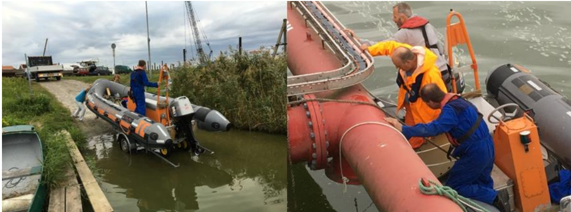
Figure 7.1: The housing was installed with a Zodiac at the Den oever site
