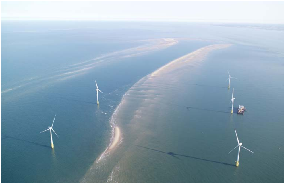
Plate 2. Aerial view of the wind-farm under construction with the jack-up barge in position (courtesy of Aerial Images Ltd).
