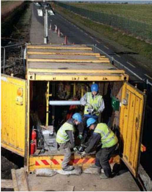
Figure 2b.7: Image of a HV cable jointing shack
