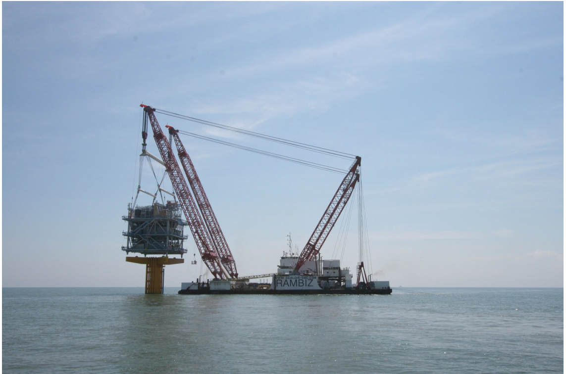
Figure 2a.12: Installation of offshore substation at the London Array Offshore Wind Farm
