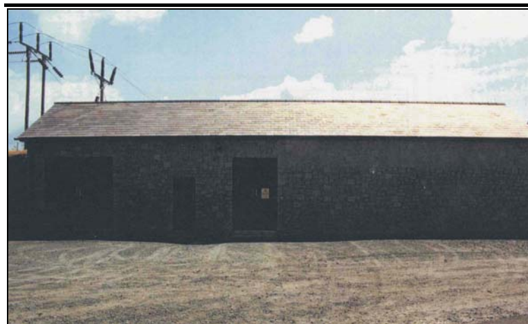
Figure 4.2 Photographs of a Typical Substation
