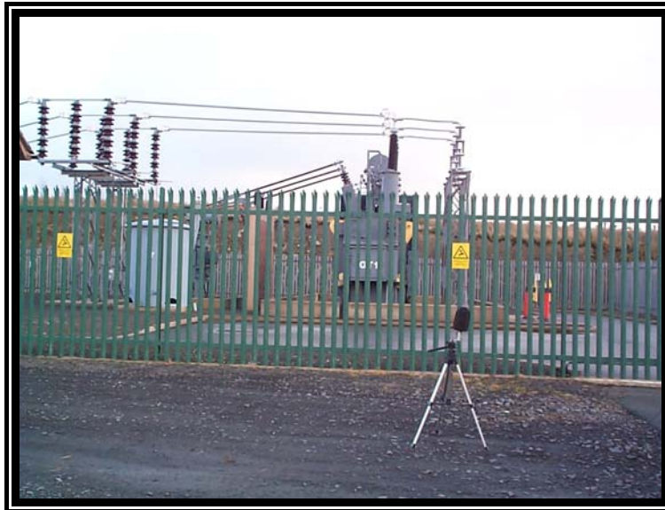
Measurement Position for Substation Noise Measurements
