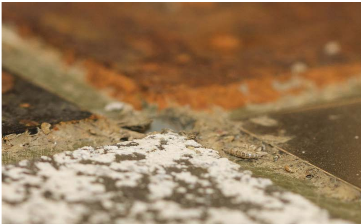
Figure 4.2 – Fouling and sediment deposition along edges and in crevices
