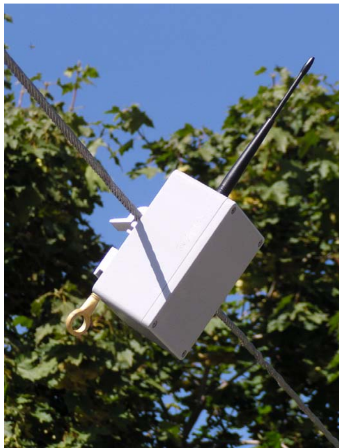
Figure 3. Bird Strike Indicator (BSI) sensor installed on a power line
