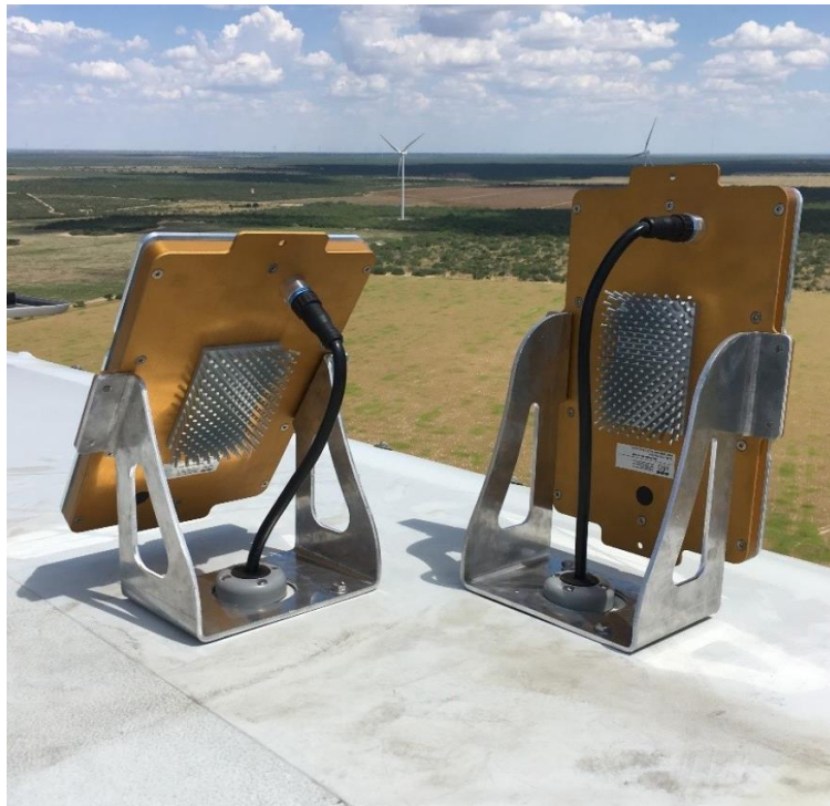
Figure 12. Two installed acoustic deterrents on top of a wind turbine nacelle at Duke Energy's Los Vientos facility. Image by Will Ramirez (2019).
