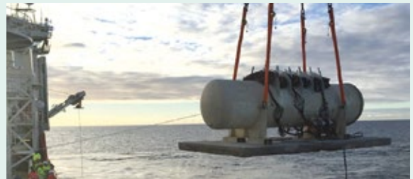
Seabased wave energy converters (top) and low voltage marine substation (down) under installation at Sotenäs. Courtesy: Seabased
