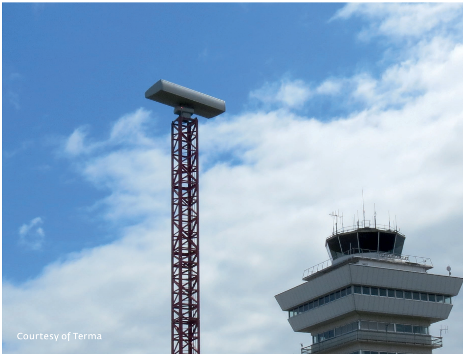
Test installation of SCANTER 4002 radar, CPH Airport
