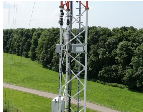
Fig. 8. Photo of the field installation at WINSSENT.
