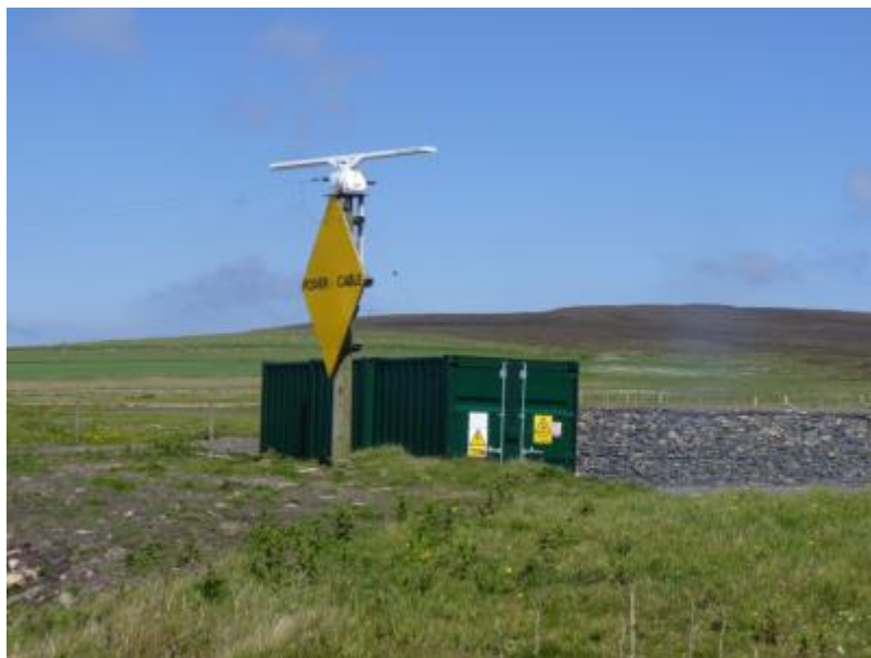
Figure 3: Marine X-band radar system installed at EMEC electricity substation
