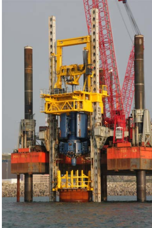
Figure 46: Operation of a marine vertical drilling machine off the coast of Flamanville, Normandy. The outfall installation of a nuclear power plant was founded in strong bedrock formations by drilling 63 m deep with drill head diameters of 5.85 m and 6.35 m (source: Fugro Seacore Ltd. )
