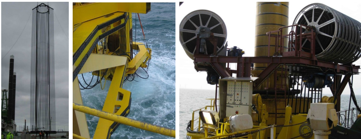
Figure 12: Little bubble curtain of vertical hoses (SBC of MENCK/BARD ). Concept tested at OFT 1 (left and middle, see text) and improved concept for OFT 2 (right) (source: STEINHAGEN 2012)
