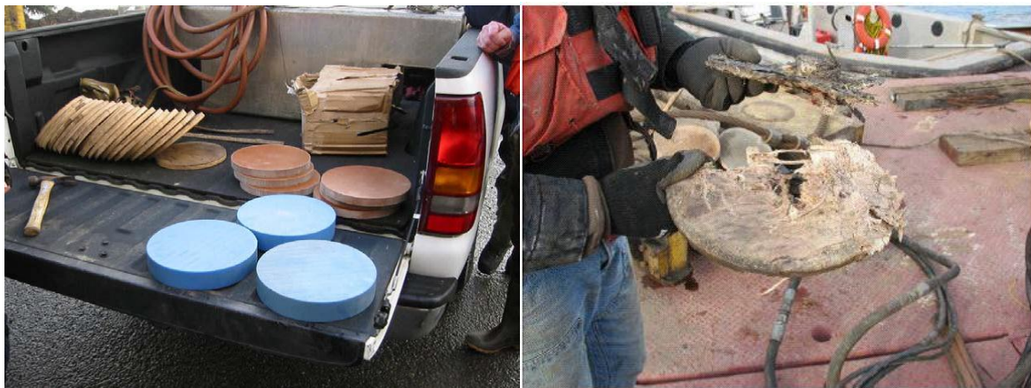
Figure 34: Piling cushions tested in the experiments by the Washington State Department of Transportation before being used (left), and fractured and compressed plywood piling cushion after being used (right) (source: LAUGHLIN 2006)
