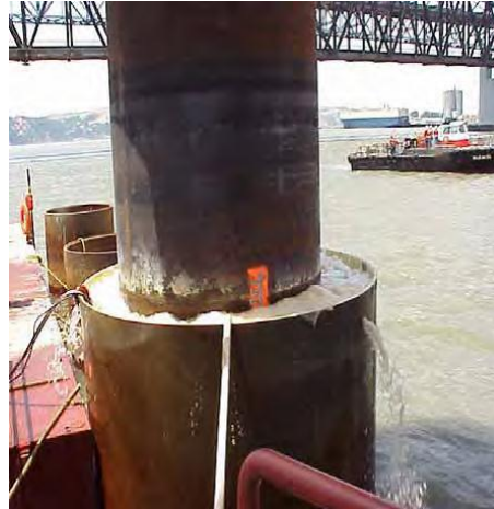
Figure 16: Isolation casing with additional bubble curtain between pile and isolation casing during piling of a 2.4 m pile at the Benicia-Martinez Bridge, California (source: CALTRANS 2007)
