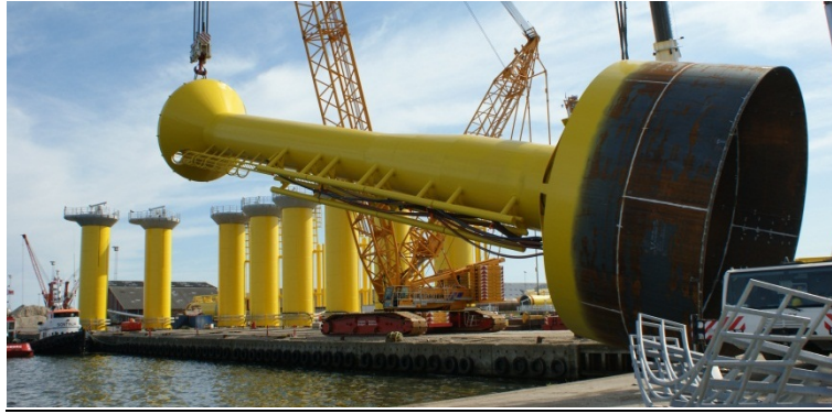
Figure 66: Bucket foundation of a mobile met mast for the OWF Horns Rev 2 during erection in the port (source: LEBLANC et al. 2009)
