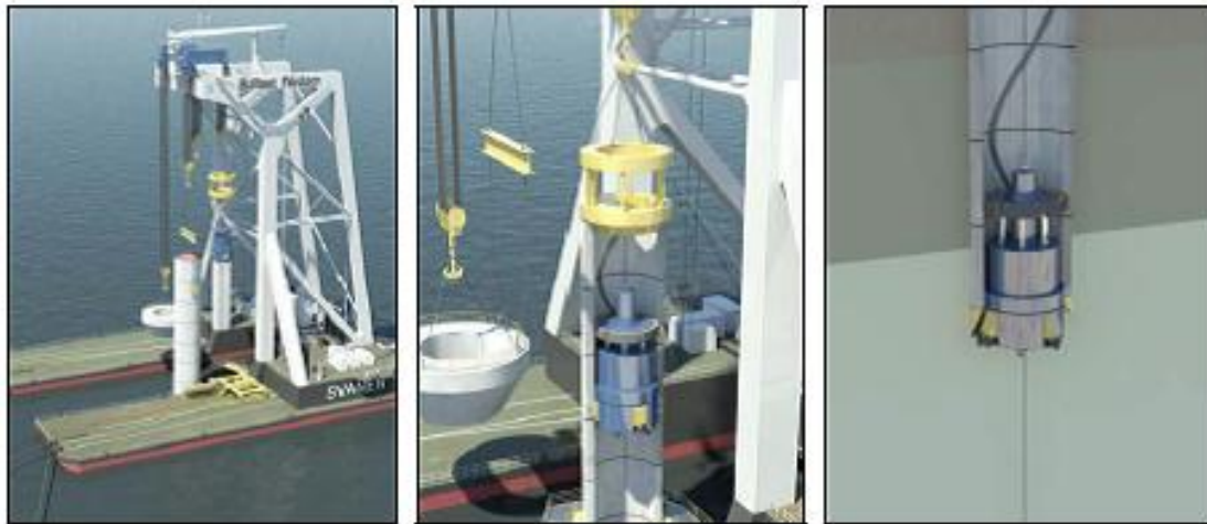
Figure 43: Drilled concrete monopile concept of Ballast Nedam : positioning (left), drill head before installation within the monopile (middle), drilling operation and penetration of the monopile (right) (source: VAN DE BRUG 2011)
