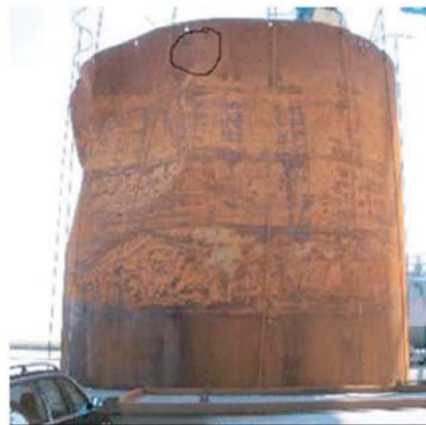
Figure 65: Deformed bucket foundation of an Enercon E 112 wind turbine near Hooksiel (source: IBSEN & NIELSEN 2007)
