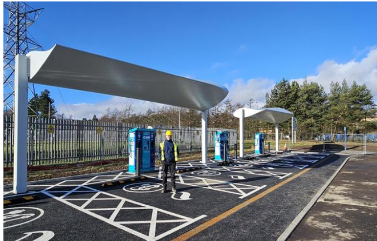
Figure 10: EV charging hub in Kingsway West, Dundee, with canopies made from decommissioned blades by ReBlade.
