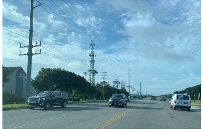
Transmission line and communications tower in Kill Devil Hills.
