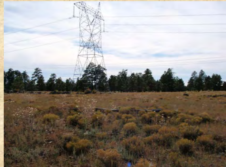
Above: Existing Western Transmission Line, Potential Interconnection Area. Left, an existing 345kV switchyard
