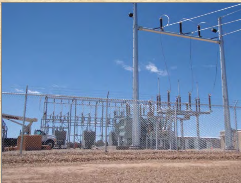
Above: Typical Step-up Substation
