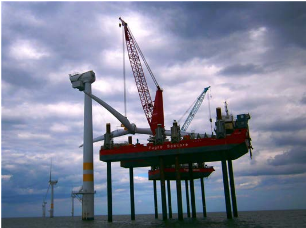
Figure 6.3. Example of jack-up platforms (Fugro Excalibur and Deep Diver)
