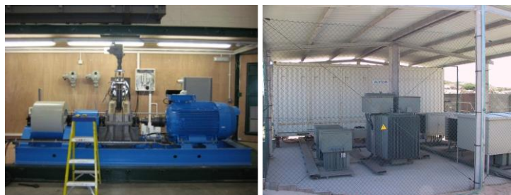
Oyster – 315kW Pelton turbine, flywheel and induction generator (left photo: Aquamarine Power) and AWS - 6MVA AC/AC Converter, M.V. Switch Gear and Power Transformers (right photo: Teamwork Tech. B.V.)
