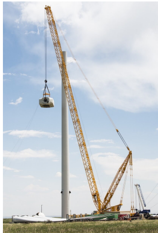
Figure 12. Crews lower the nacelle as part of the decommissioning of the 3-MW Alstom wind turbine at NREL's National Wind Technology Center. Photo by Dennis Schroeder. NREL 51733
