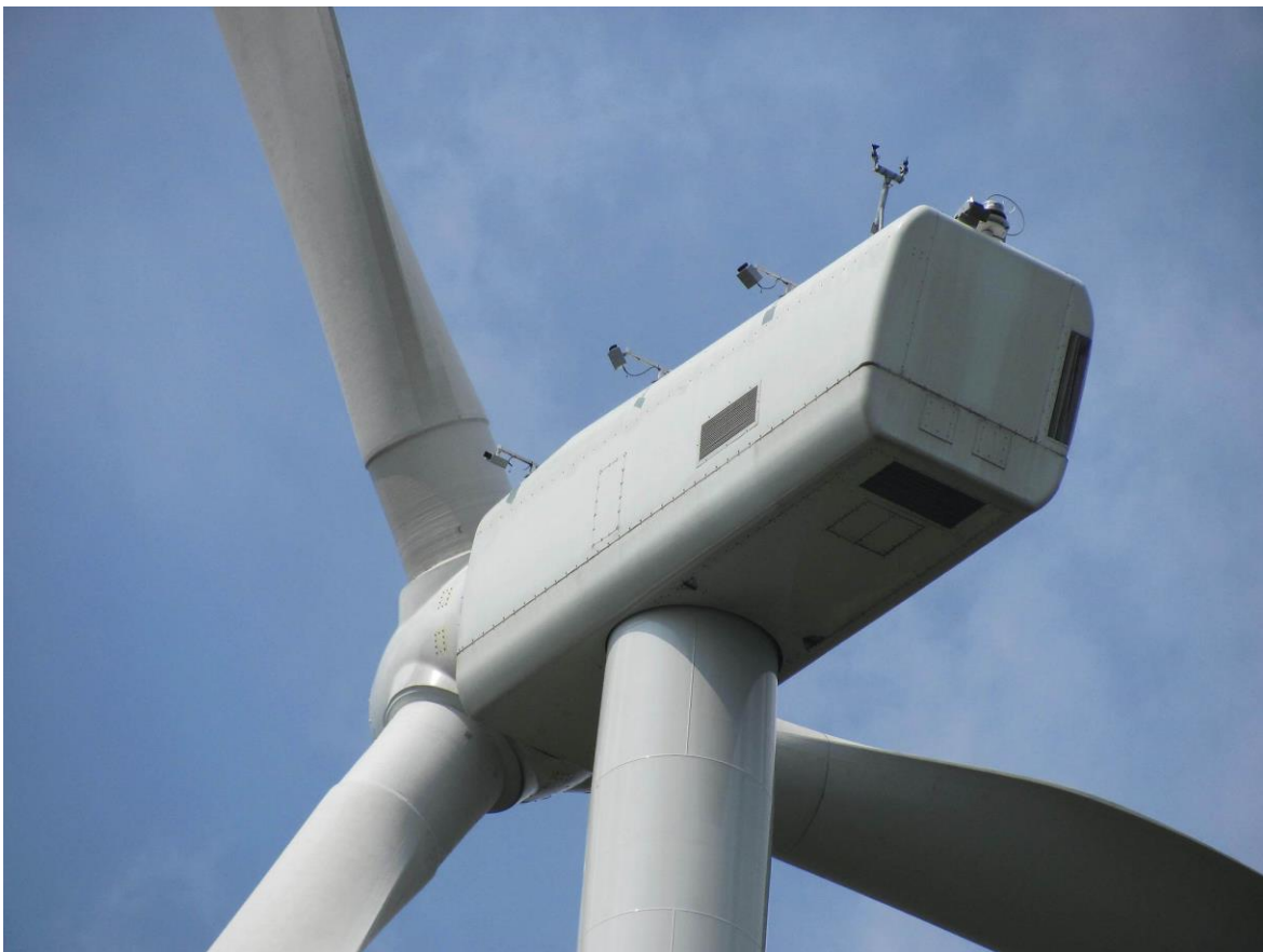
Ultrasonic acoustic deterrents mounted on the side of the nacelle (photo by E. B. Arnett)
