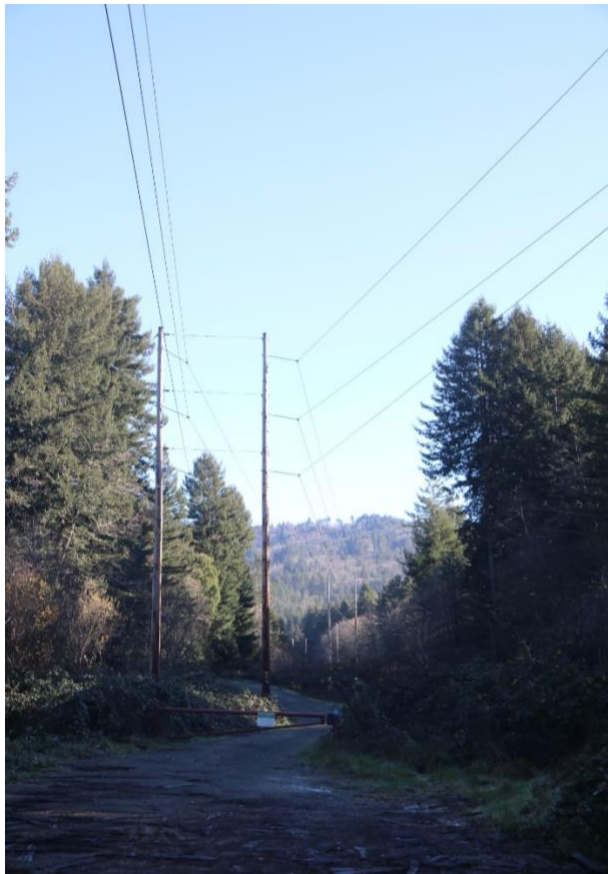
Figure 3. Two parallel 115-kV transmission lines run northeast from Crescent City toward Grants Pass where they connect to 500-kV lines.
