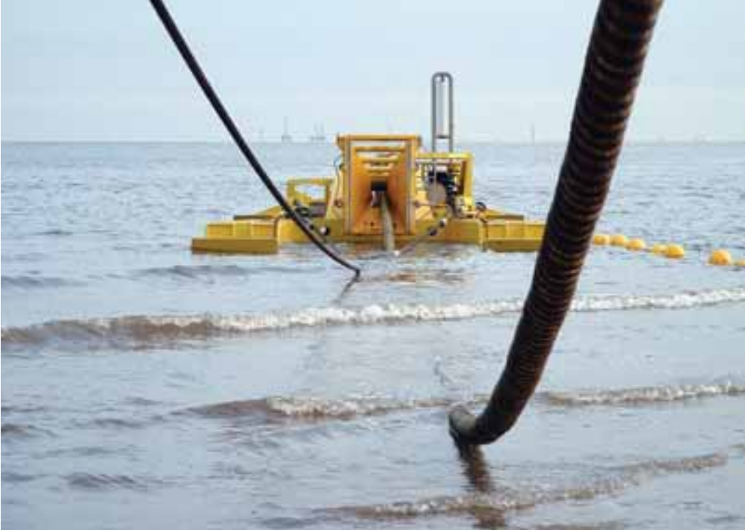
Figure 3.14: Sea Stallion 4 Cable Plough Burying North Hoyle Export Cables up the Beach
