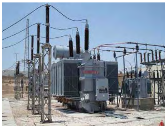
Figure 4.14 Example outdoor 33kV substation
