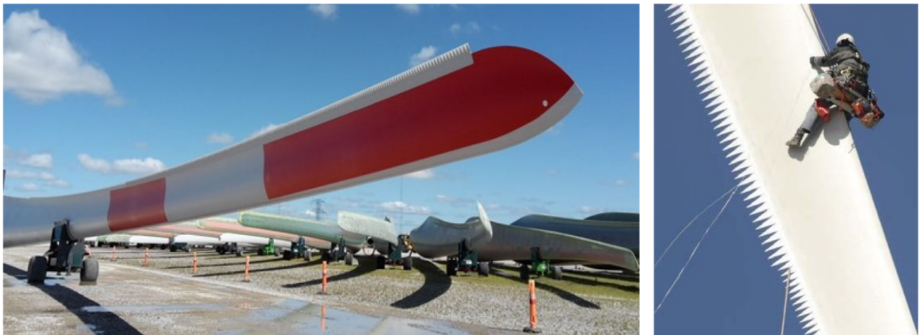
FIGURE 3 Serrations mounted on wind turbine blades (Source: Siemens Gamesa Renewable Energy (Oerlemans et al., 2009)).
