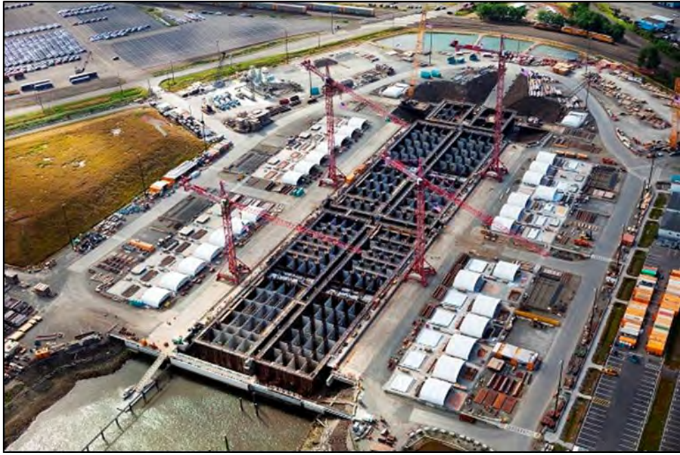
Figure 5-2. Grays Harbor Casting Basin for SR 520 Pontoons (Washington State Department of Transportation 2013)
