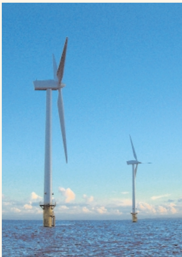
Blyth offshore wind farm
