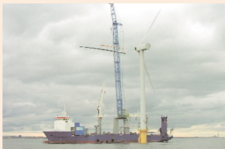
Blyth offshore wind farm
