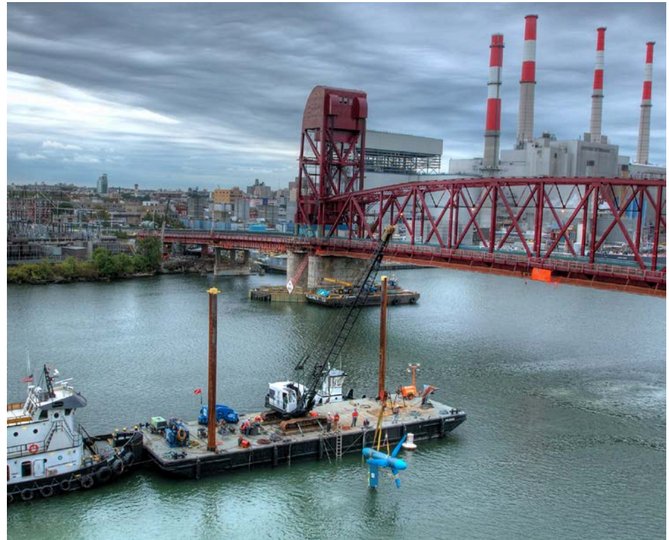
Verdant Power RITE Project (East River; New York, NY)
